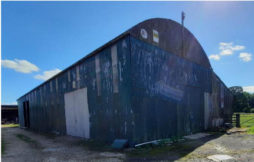
Figure 2. Main Barn 541 m 2 - to be extended and become the Distillery and Visitor Centre
