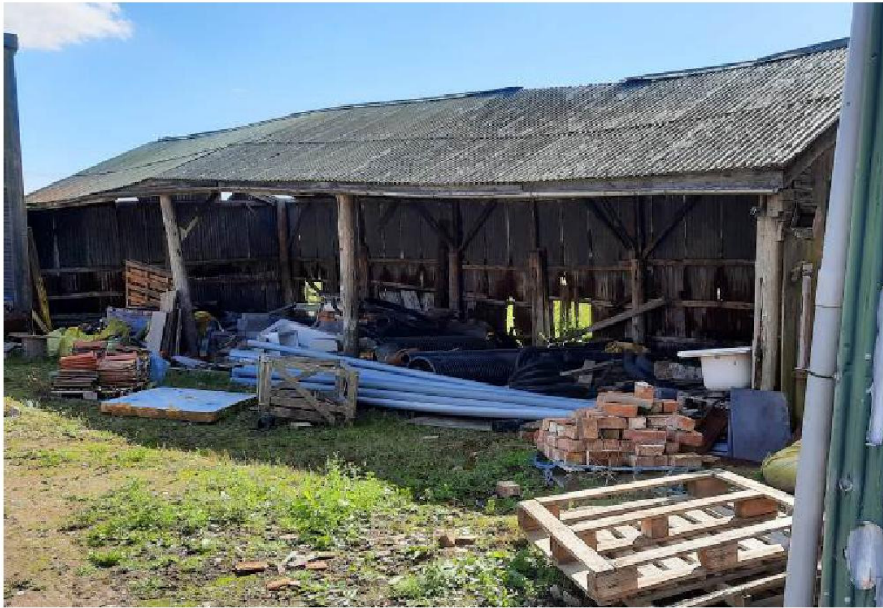
Figure 6. Rear Dilapidated Barn 95 m 2 to be removed and replaced and become the Plant Room and part of Store 2
